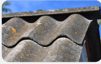
Asbestos roof sheets
