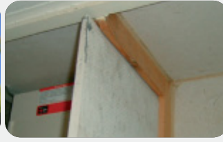
Asbestos insulation board
